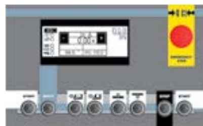
CONTROL PANEL: MITSUBISHI
